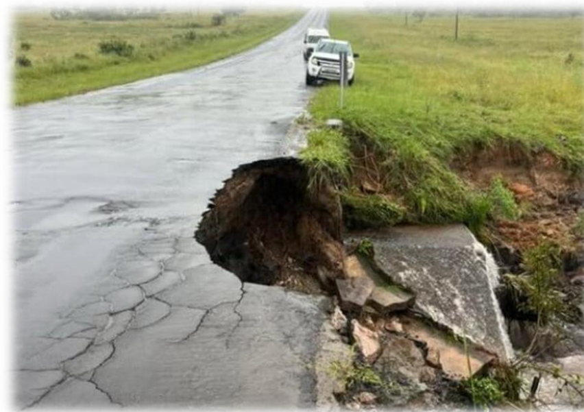
IMAGE 8: INFRASTRUCTURE DAMAGE CAUSED BY FLOODING
